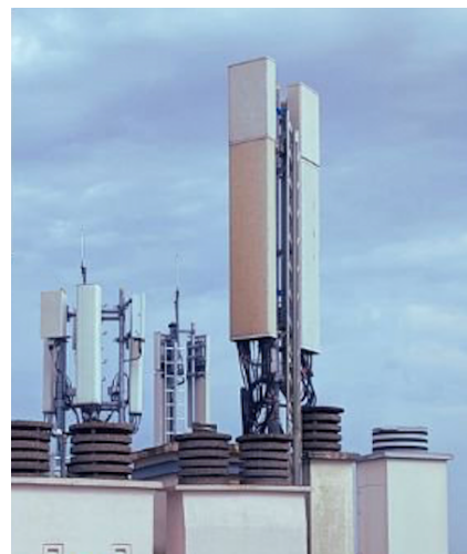
Figure 35 : type de pose d'antenne-relais non acceptable
